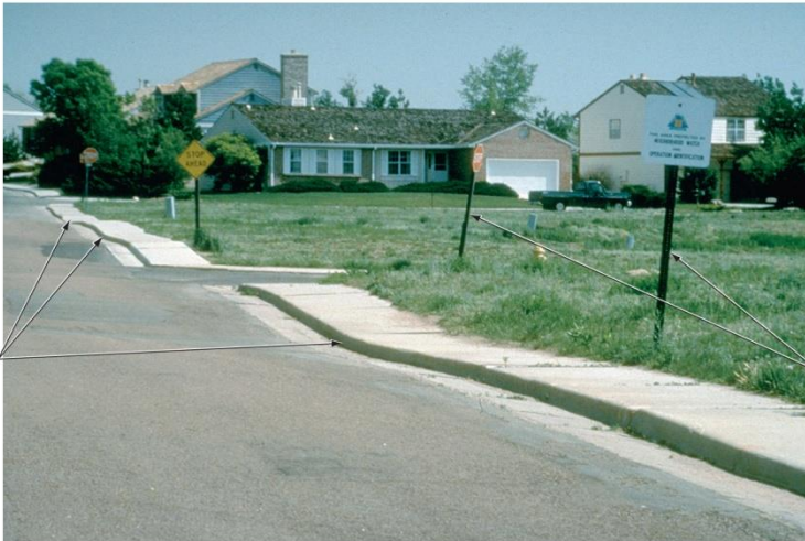
Depressions in road and sidewalk
