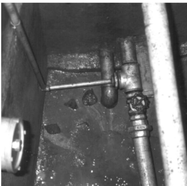
Easy accessible operation chamber – well maintained
